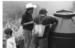
Guatemala Mission - mountain rainwater retention system
