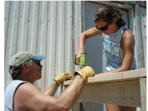
Melissa Rink and Ted Brown put the finishing touches to a new front porch and stairs.
